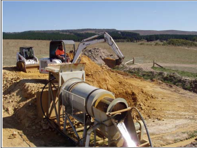
Processing Plant - Scrubber unit- Shiralee T2 prospect ©
